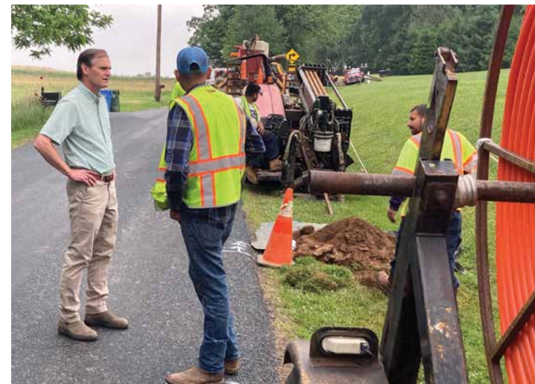
Billy Boniface, left, chief advisor to County Executive Barry Glassman, talks with a representative of ThinkBig, which installed the first underground fibers as part of its partnership with Harford County to bring high-speed internet service to homes and businesses in the northern part of the county.
